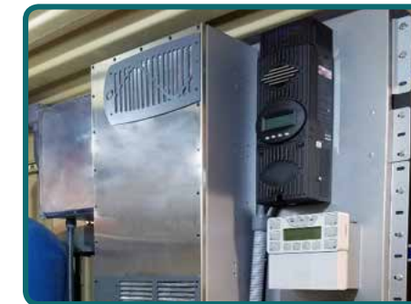
Control Panel and PLC on MWPS-4000
