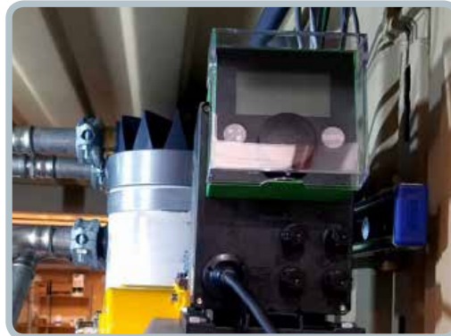
Chlorine Dosing Pump on MWPS-4000
