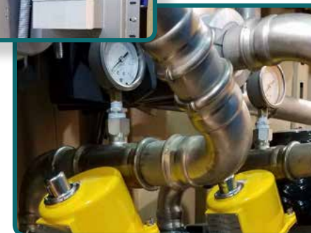
Automated Backwash Valves on MWPS-4000
